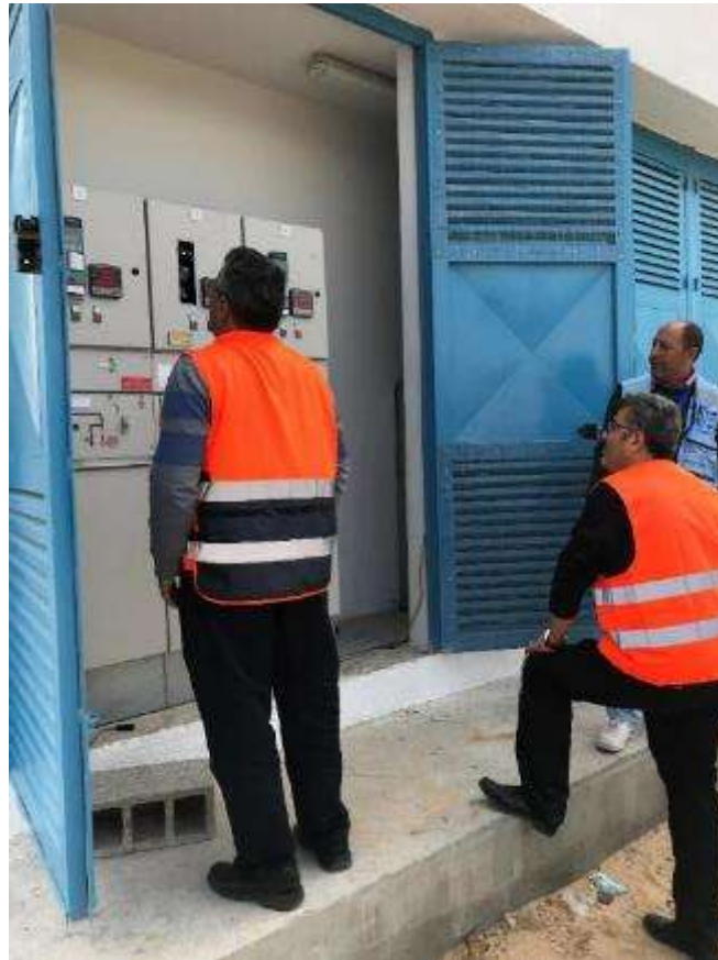
Fig. 14: Field Audit Team Evaluating a Transformer
