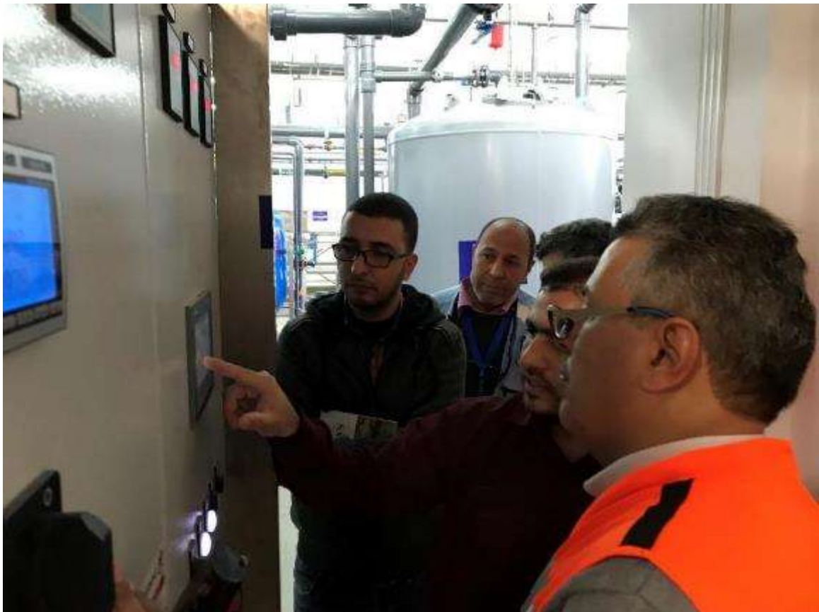
Fig. 12: Field Audit Team Evaluating the Desalination Plant
