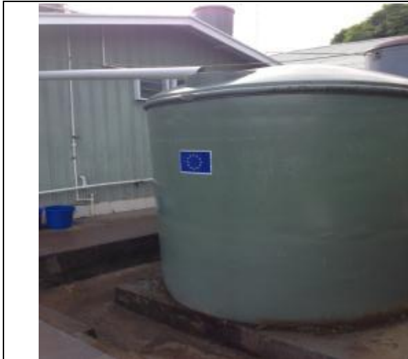
9 May 2019. TCA base, rainwater harvesting tank (EU funds).
