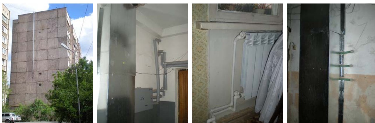
Figure 4: Pictures from Avan district of Yerevan, May 2008. a) Multi-apartment panel building with exhaust chimney from gas heater installed in one apartment (not financed by the project!), b) New 'risers' installed in stairwell with meter and start of network, c) New radiator in apartment, d) New 'riser' ready to accept connection if the apartment owner decides to join the scheme (photographs Grant Ballard-Tremeer).
