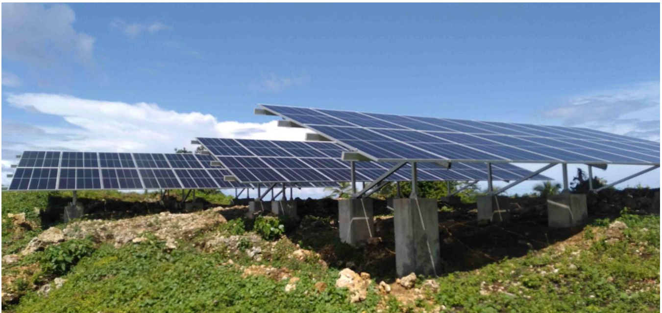
Figure 3: Solar panels mounted in Rokera
