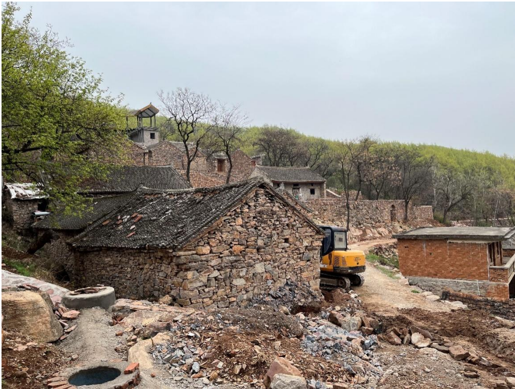
The evaluation team visited the cultural tourism construction site in Stone Village
