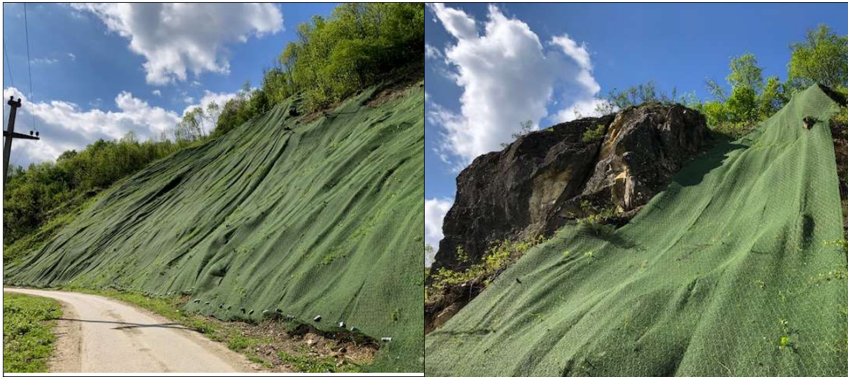
Senokos-Lomnica – site 1: road protection: net not fixed to the ground with staples
