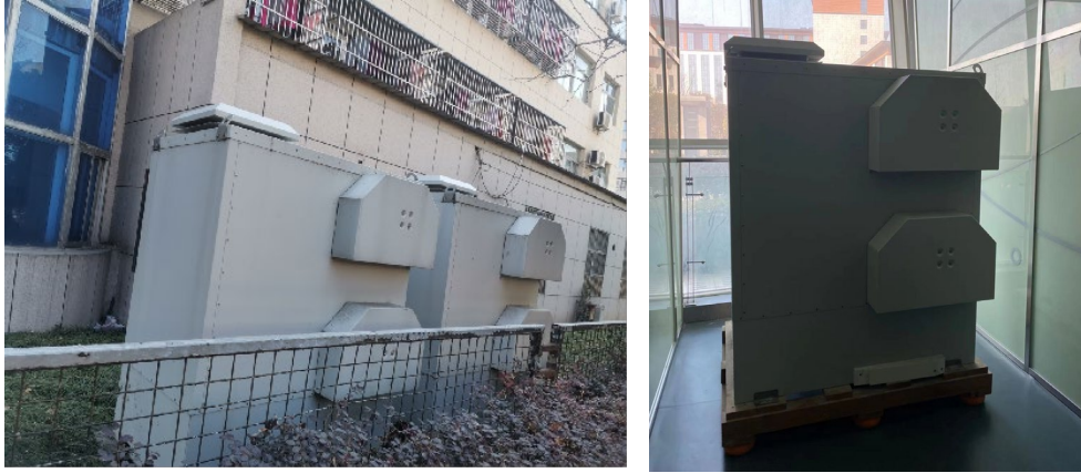
Figure 9 Backup Power System
