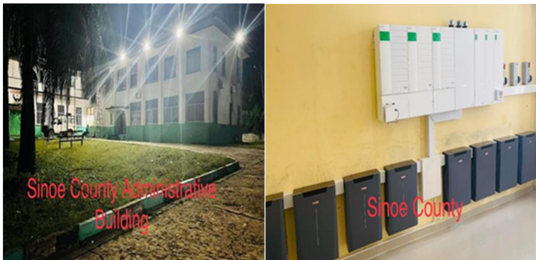
Sinoe county administrative building after renovation and installation of solar lighting for lighting and powering computers
