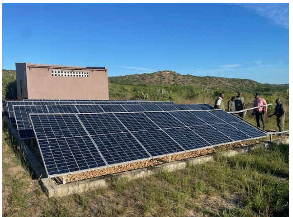
Solar panel systems in PNR
