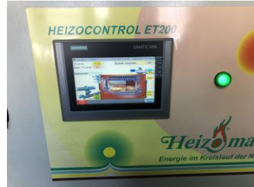
Biomass control panel
