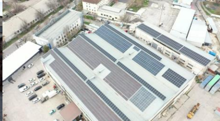
Aerial view of solar array
