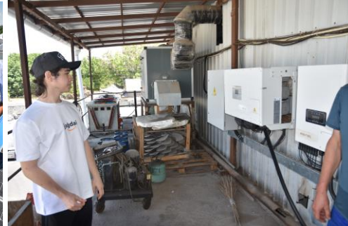
Control panels of solar array
