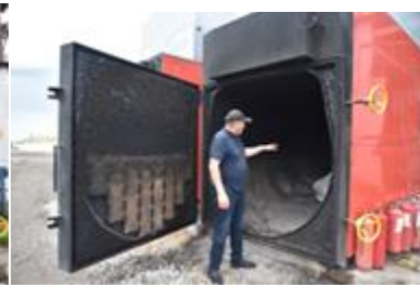
Interior of boiler
