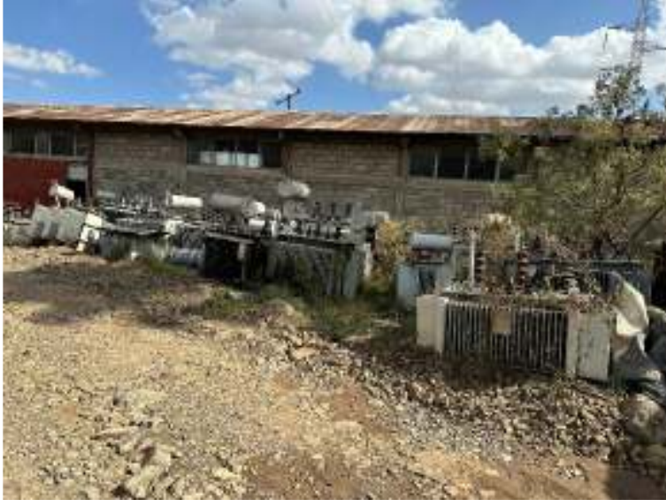
PCB-contaminated Equipment at Ethiopian Electric Power (EEP)
