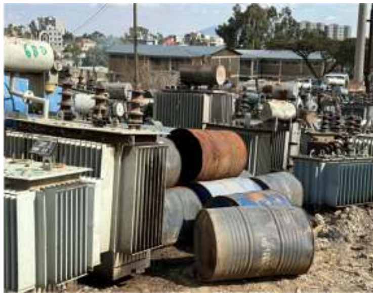
PCB-contaminated Equipment at Ethiopian Electric Power (EEP)
