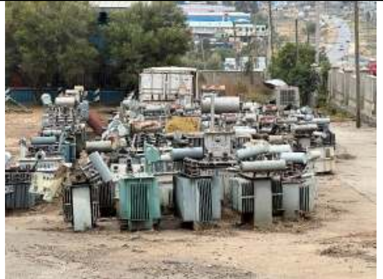
PCB-containing Equipment at Ethiopian Engineering Group (EEG)
