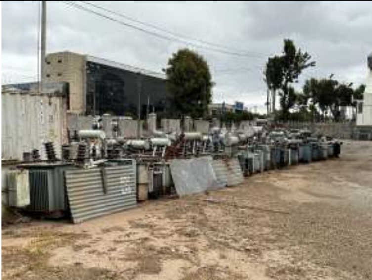
PCB-containing Equipment at Ethiopian Engineering Group (EEG)
