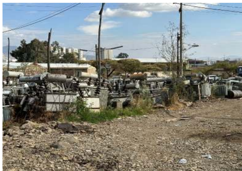
PCB-contaminated Equipment at Ethiopian Electric Power (EEP)
