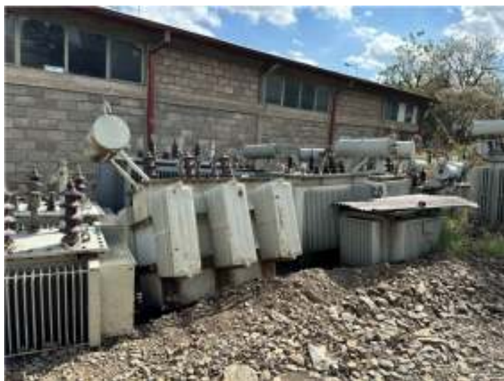
PCB-contaminated Equipment at Ethiopian Electric Power (EEP)
