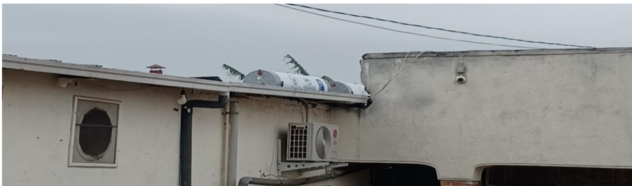
Solar-powered water heaters at Binya Bakery Limited, Gasabo District
