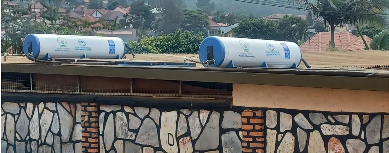
Solar-powered water heaters at New Vision Bakery, Kicukiro District
