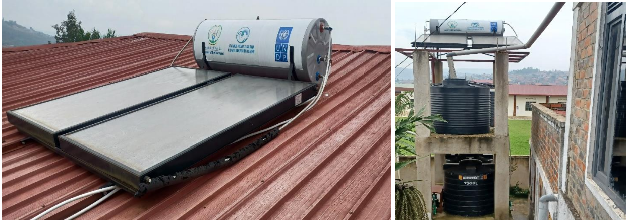
Solar water heater (left) and water tank system (right) at Alegria Inn, Kamonyi District
