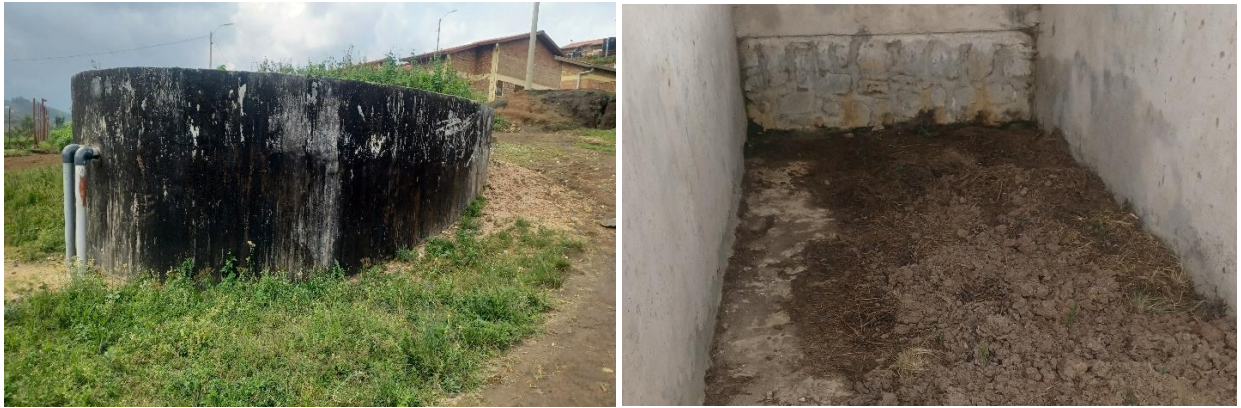
From left to right: water tank and compost pit at Kivugiza IDP village, Nyaruguru District
