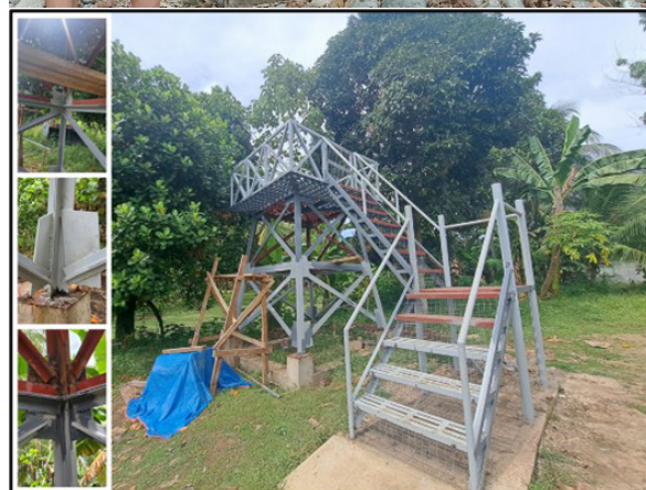
Ongoing construction of the water system in Barangay Kilangan, Pagalungan in Camp Badre (Photos by Michael Jess Lapid).
