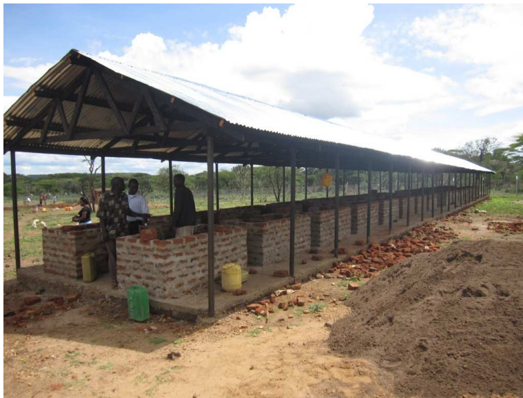
Nakiloro ‘border market’ under construction: creating shared interests and community goods- linking infrastructure, livelihoods, economic activity, cross-border collaboration and security
