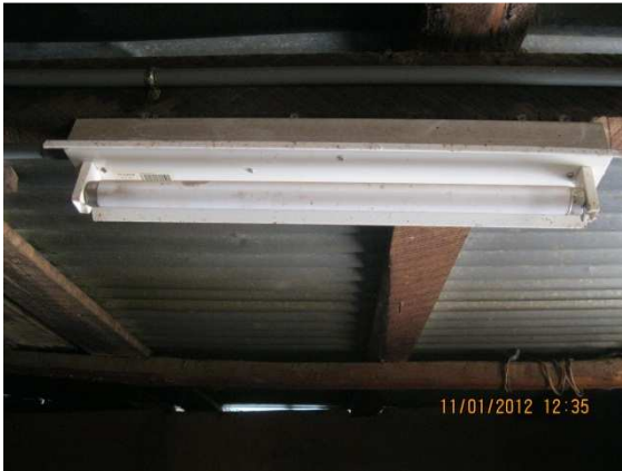
Luminaria instalada a 12 VDC
