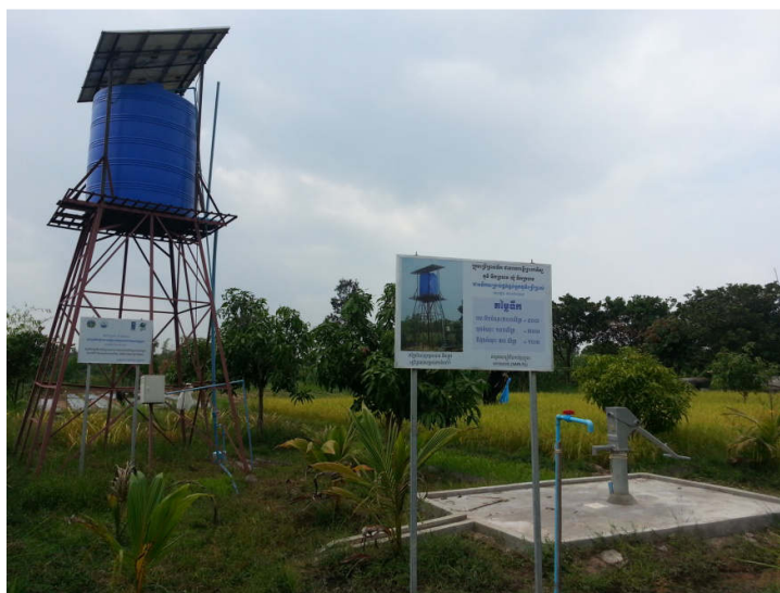
Field visit, solar water pump and tank at NAPA FU beneficiary place in Teuk Krahorm Commune, Preah Vihear Province, 28 October 2013
