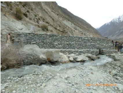
Photo of completed first portion of protection wall at village Chira Bari Bar Bagrote
