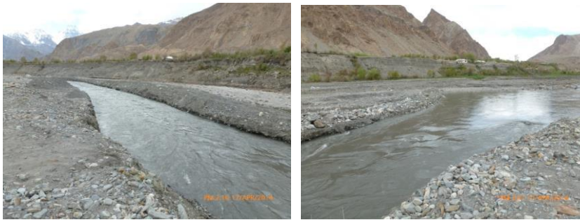
Excavated river channel on the left side and diversion dike on right side for Chitral River at Shogram Payen village Bindo Gole
