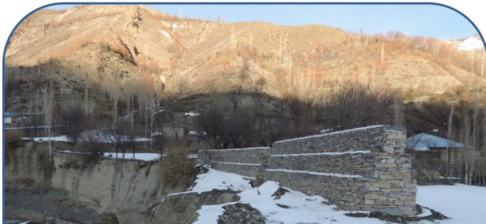
Figure 6 Climate Change Adaptation structures as constructed to reduce the vulnerability of the exposed communities. Note the construction of gabion walls both at the foot slope, aimed at resisting
