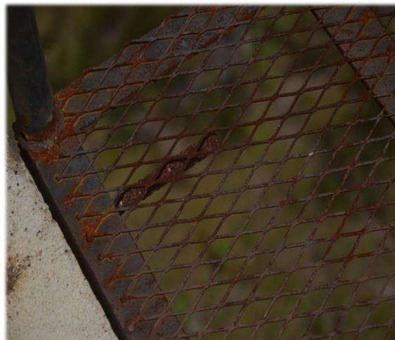
Figure 4: Platform and stairway at the highest level of a CLIFOR-funded fire observation tower showing high levels of rust and unsafe conditions.
